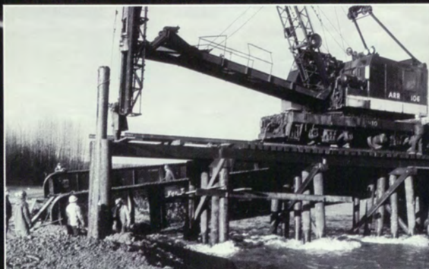
Montana Creek Bridge was damaged in October when severe flooding washed out bridges and portions of track, halting most services for two weeks.
