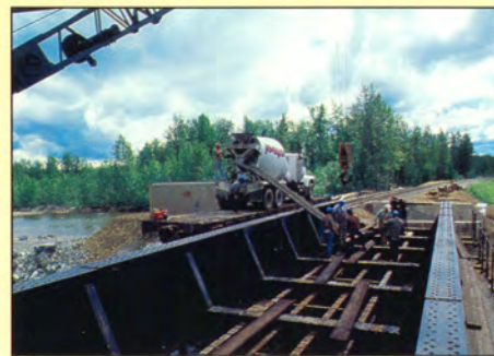
The original 80-foot span on the Montana Creek Bridge, damaged in the 1986 flood, was salvaged and a 60-foot span added in 1987 to increase the water flow capacity of the bridge and reduce future risk of flood damage. The work was performed during live track conditions by Building and Bridge crews.
