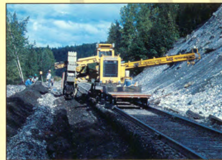
During 1987 summer work programs, Maintenance of Way employees used an undercutter to remove ballast damaged in the October 1986 flood. Specially designed for railroads, the undercutter lifts the rails and ties then digs out the ballast. Nearly 17,000 feet of rail were undercut and nearly 9,000 yards of ballast replaced in locations from Seward to Healy.
