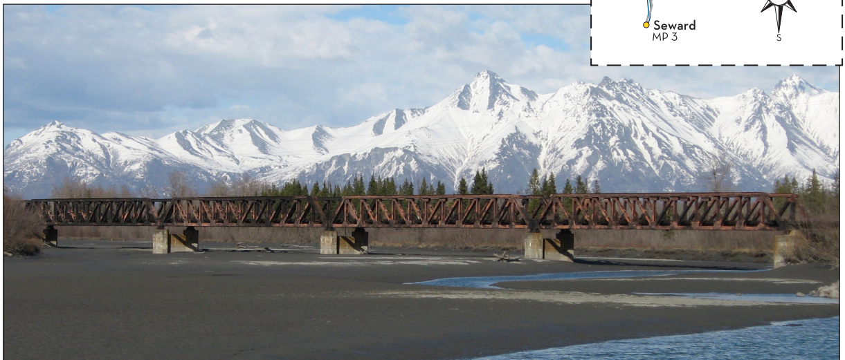
The pony truss bridge at ARRC milepost 147.5 spans the North Channel of the Knik River.
