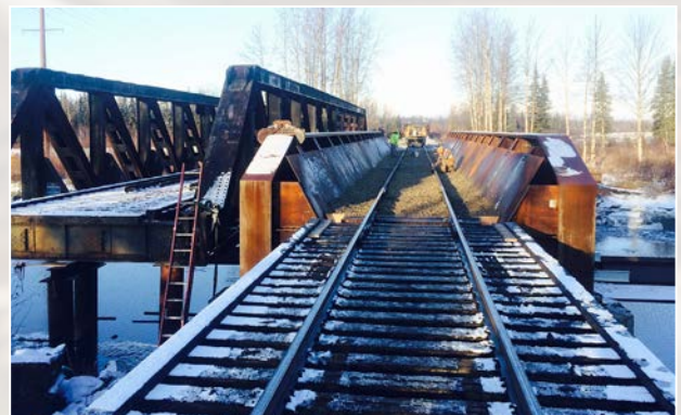
A new thru-girder bridge replaces the old military pony truss bridge (left) crossing Matanuska Flood Plain waterways.
