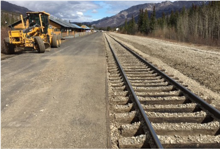
The main line track is realigned to replace the siding next to the Denali Depot's passenger platform.
