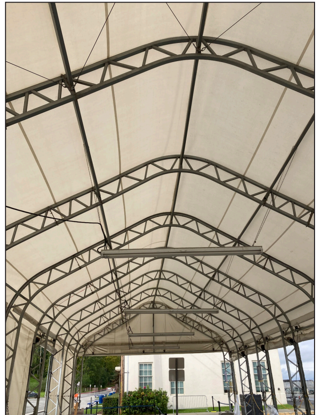
The Anchorage Historic Depot's structure is fortified with a sturdy frame. The depot's baggage shelter cover is reaching the end of its useful life and must be replaced.
