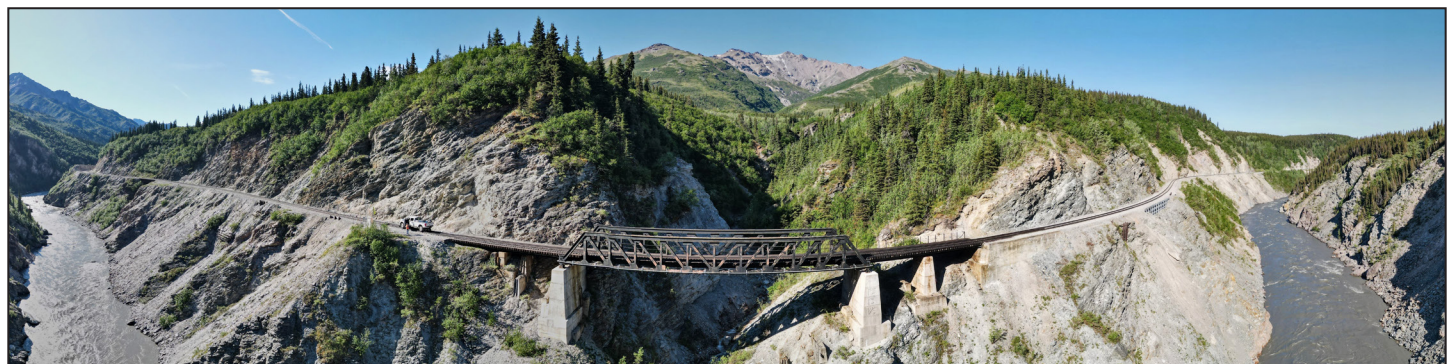
A panoramic view of Bridge 354 shows the surrounding steep banks of the Nenana River.
