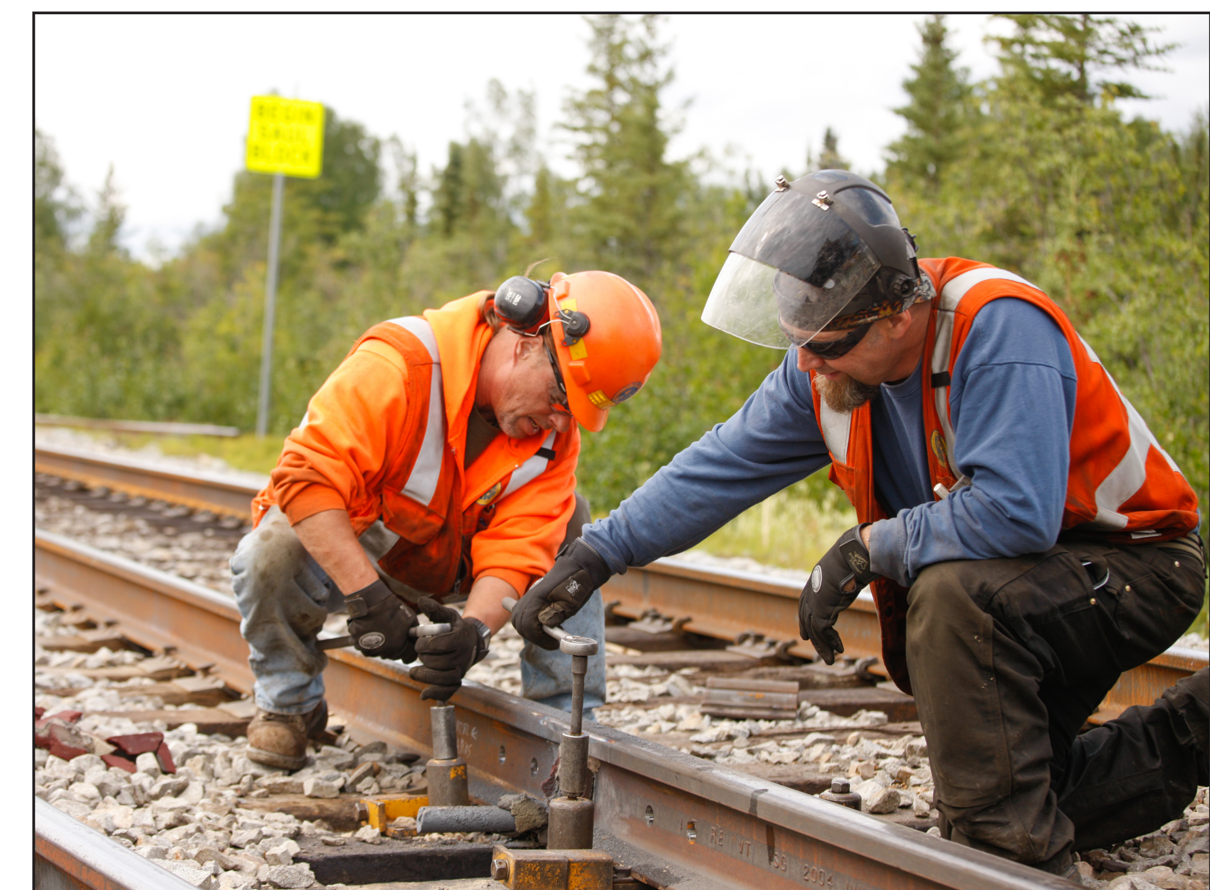
Controlled vegetation helps to minimize trip, slip and fall hazards to employees who work along the track.
