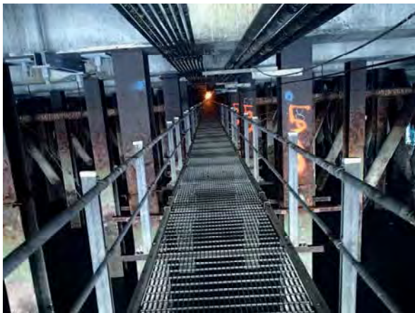
Catwalk and Electrical Conduit Under Dock
