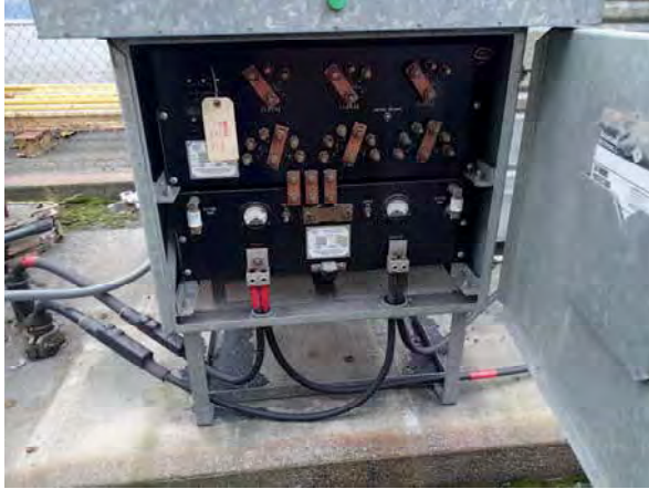
Typical Air Cooled Rectifier
