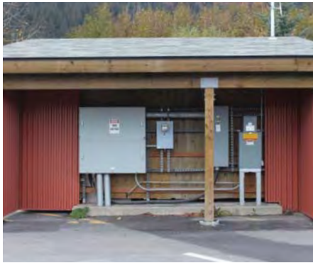
Electrical Train Storepower
