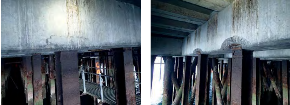
Cast-In-Place Concrete Pile Cap with Local Spalling at Pile Embed.
