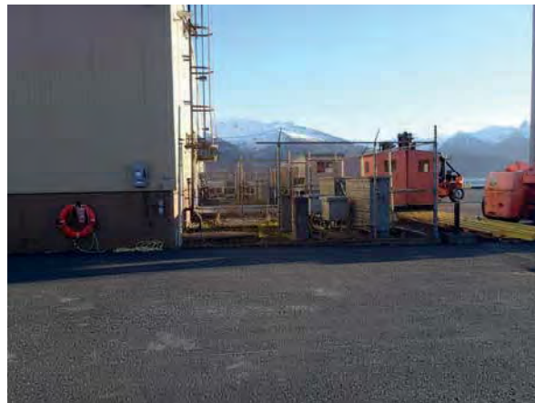
CP Rectifiers Near Building
