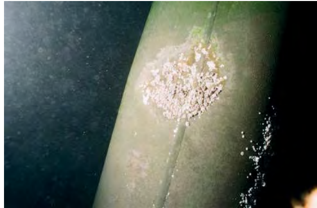
Small Dent in Dolphin Pile
