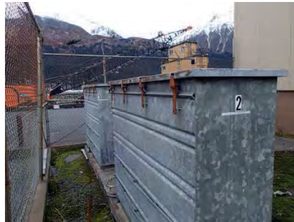
Abandoned Oil Cooled Rectifiers
