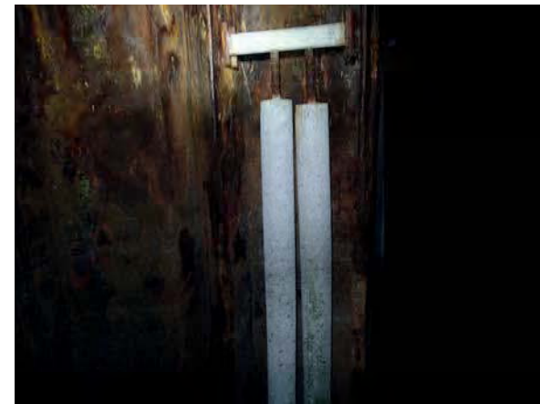
Sacrificial Anodes Near Abutment
