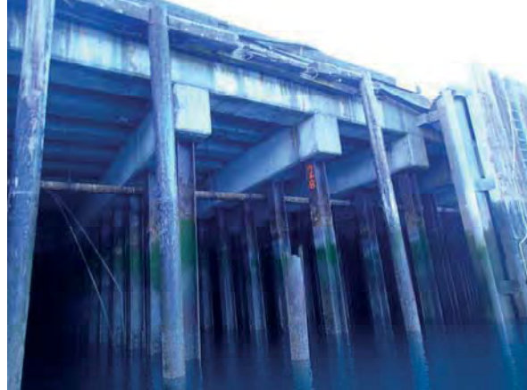
Missing and Broken Fender Piles
