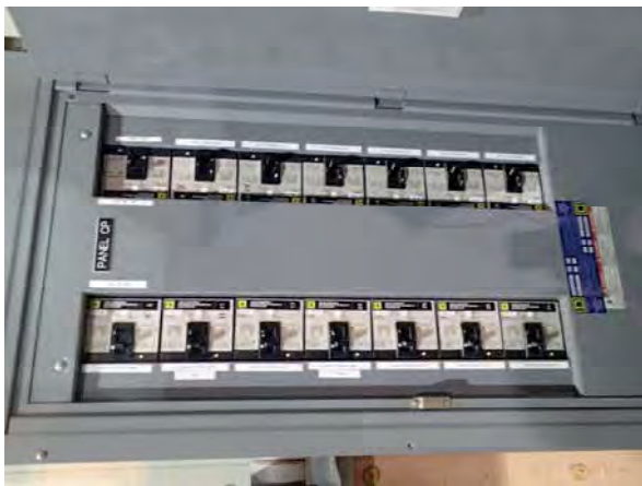
CP Breaker Panel in Terminal Building
