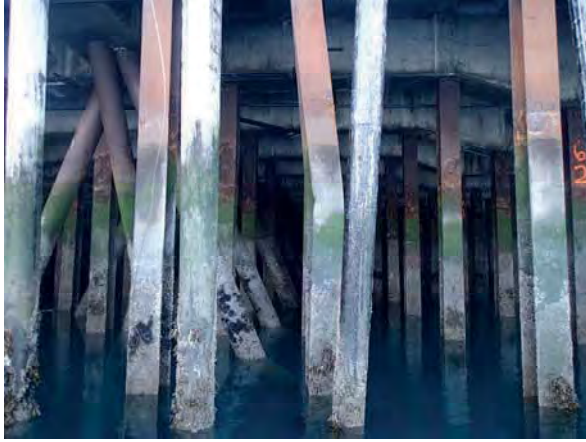
Impact Damage to Piling at Bent 63 Row 9
