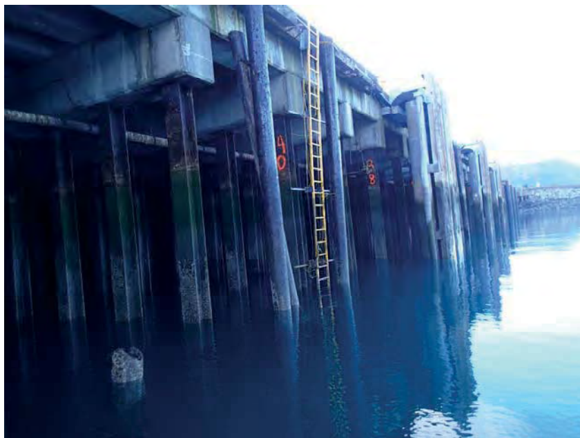
Typical ladder. Note supports detached from pile on left.
