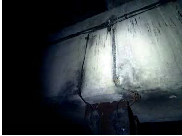
Melted Anode Wires Under Dock
