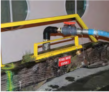
Fresh Water Service
