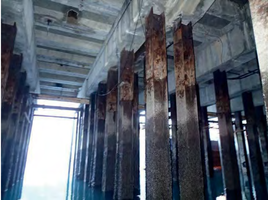
Typical H Piling. Note corrosion in the splash zone
