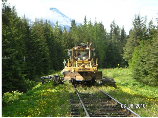
Mechanical methods on ARRC Main Track have plowed seeds and roots into ARRC ballast and shoulder section.
