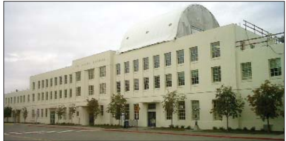
Ship Creek ITC Phase 2a work in 2010 removes utility equipment on the roof of the Anchorage Historic Depot.
