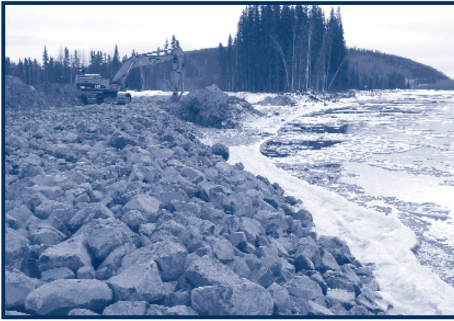
Construction on the levee requires significant rip-rap material from a local source in North Pole.
