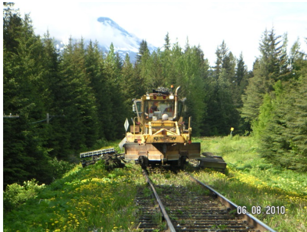
Mechanical methods on ARRC Main Track have plowed seeds and roots into ARRC ballast and shoulder section.
