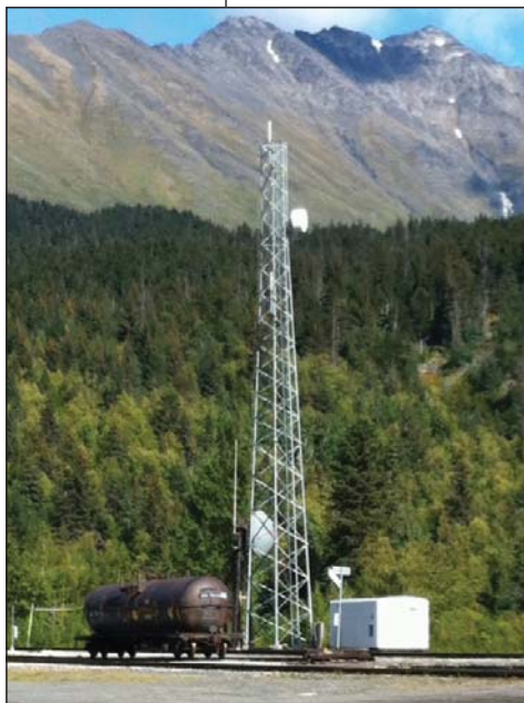
Typical ARRC Communications Site with 100-foot tower and communications shelter. Mounted antennas support microwave and radio communications.
