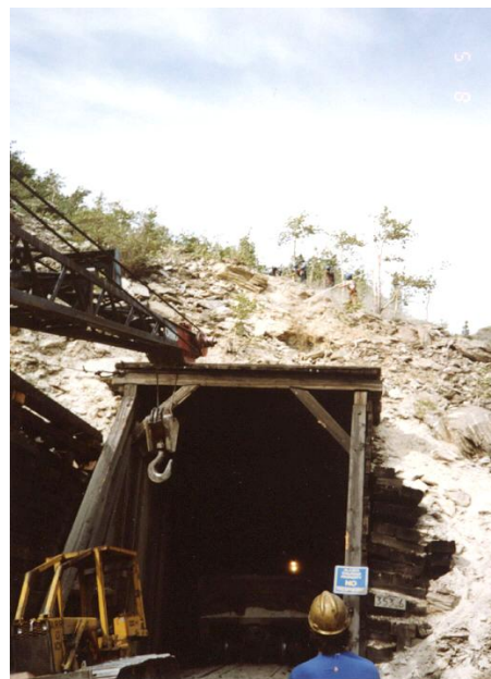
Photograph shows repairs being made after the 1992 collapse at the south end. Passenger service was disrupted for 3 days.
