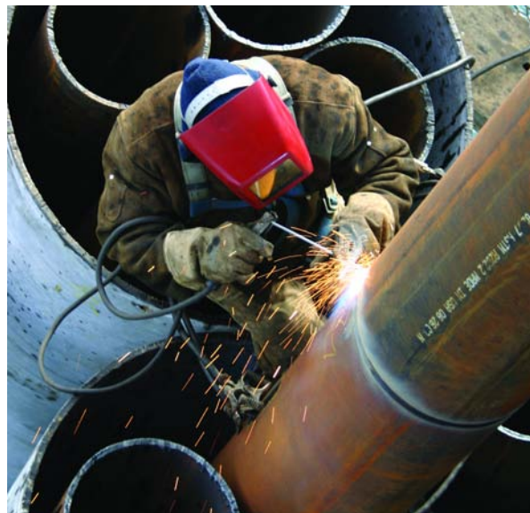
ARRC Buildings and Bridges crewman Robert Vickers works over open water on the new pylon supports for the Knik River Bridge
