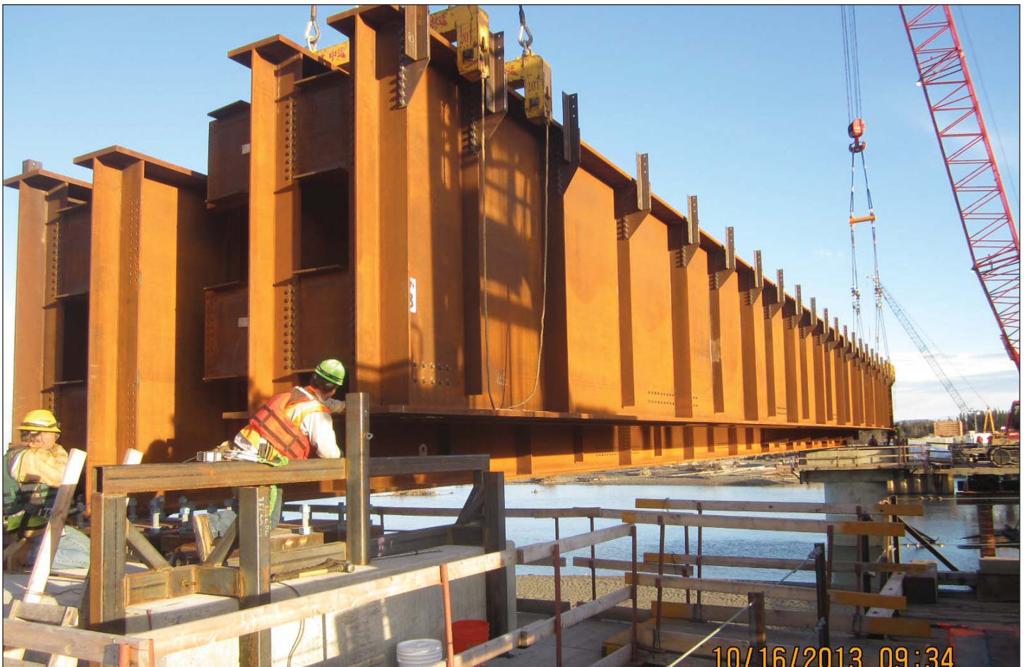
Above: The first span of 165-foot girders are placed on two piers as part of the Northern Rail Extension (NRE) Phase 1, the Tanana River bridge near Salcha. Cover top photo: Construction on the NRE Phase 1 bridge stretches across the Tanana River in early November 2013.
