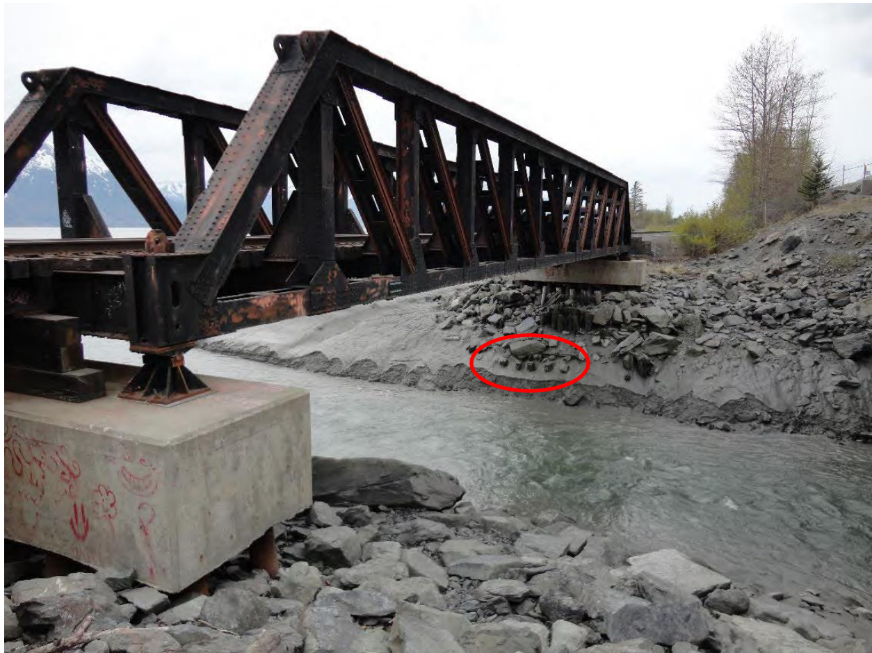
Figure 1: Creosote-treated piles circled in red.
