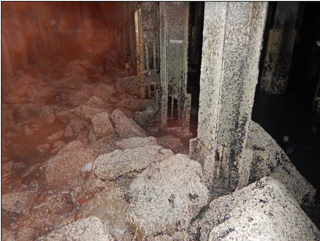
Photo 6. Typical Bent 5 and 6 Condition (Bent 5 West Side Shown)
