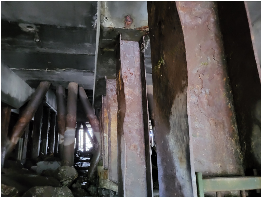
Photo 2. Typical Localized Buckling (Bent 3 Shown)
