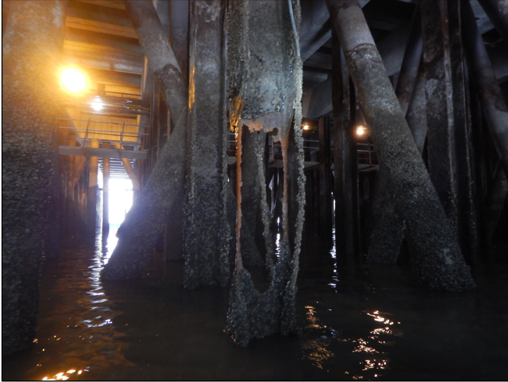
Photo 1. Typical Pile Considered Complete Loss of Section (Pile 28-21)
