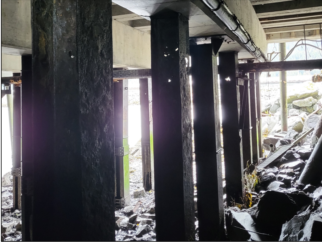
Photo 3. Typical Localized 100% Section Loss (Bent 2 Shown)
